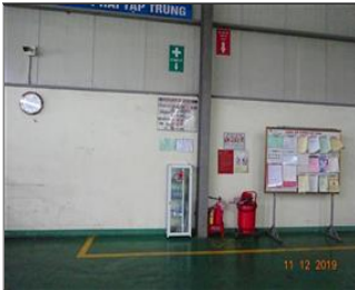
External photo(s) of the production unit(s) Fire fighting equipment were well equipped and maintained.JPG
