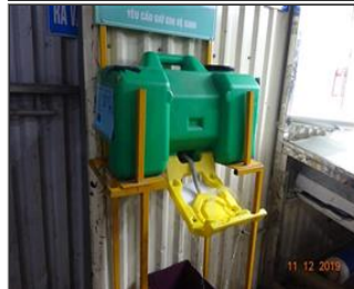
External photo(s) of the production unit(s) Eye wash station was equipped.JPG
