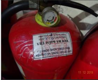
External photo(s) of the production unit(s) Fire extinguisher had been inspected by authorized department.JPG
