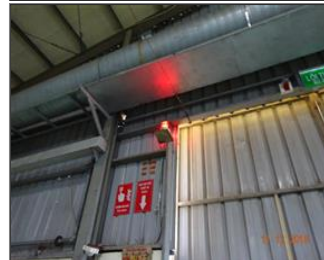
External photo(s) of the production unit(s) Fire alarm system had tested.JPG
